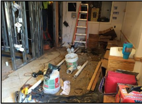
Lobby, facing electric service panels
