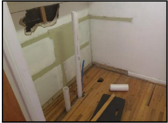
Mop sink & utility sink plumbing
